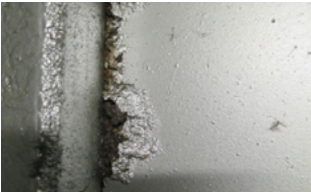
Gap corrosion on an enclosure. Through the progressing underlying rust the coating is damaged (source: OBO Bettermann)
