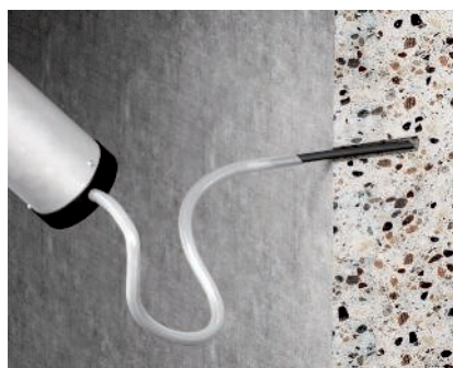
Cleaning of the drill hole Blowing-out and cleaning the drill hole with a hand-held blower or compressed air.
