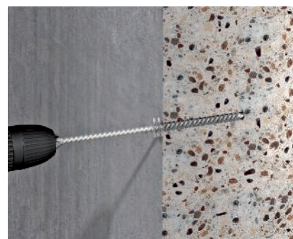
Cleaning with steel wire brush Mechanical cleaning of the drill hole with steel wire brush. The cleaning process by blowing and brushing must be carried out twice.
