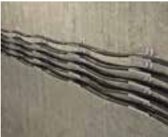
Cable support troughs
