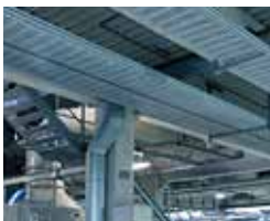
Wide span cable tray system
