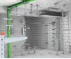
Suspended supports and brackets
