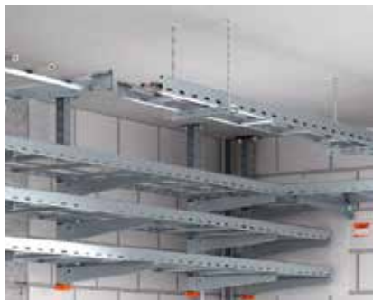
Suspended support and threaded rod suspension application Example of mounting cable ladders with suspended supports of U profiles and threaded rod suspension.
